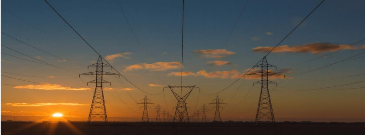
Electricity Power Lines
